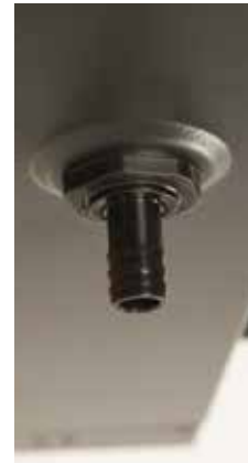
Condensation-water discharge fittings
