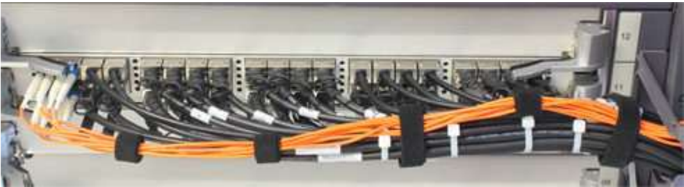
Figure 6-121 Arrangement of optical fibers and SFP+ cables
