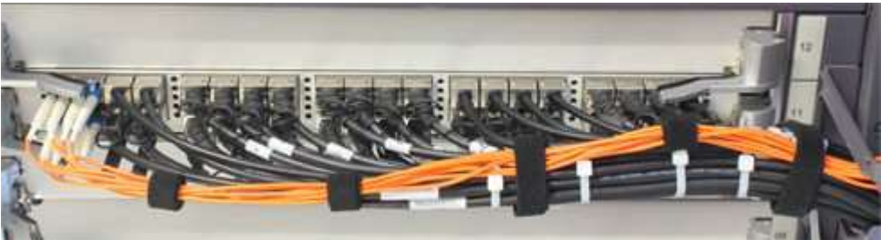
Figure 6-121 Arrangement of optical fibers and SFP+ cables
